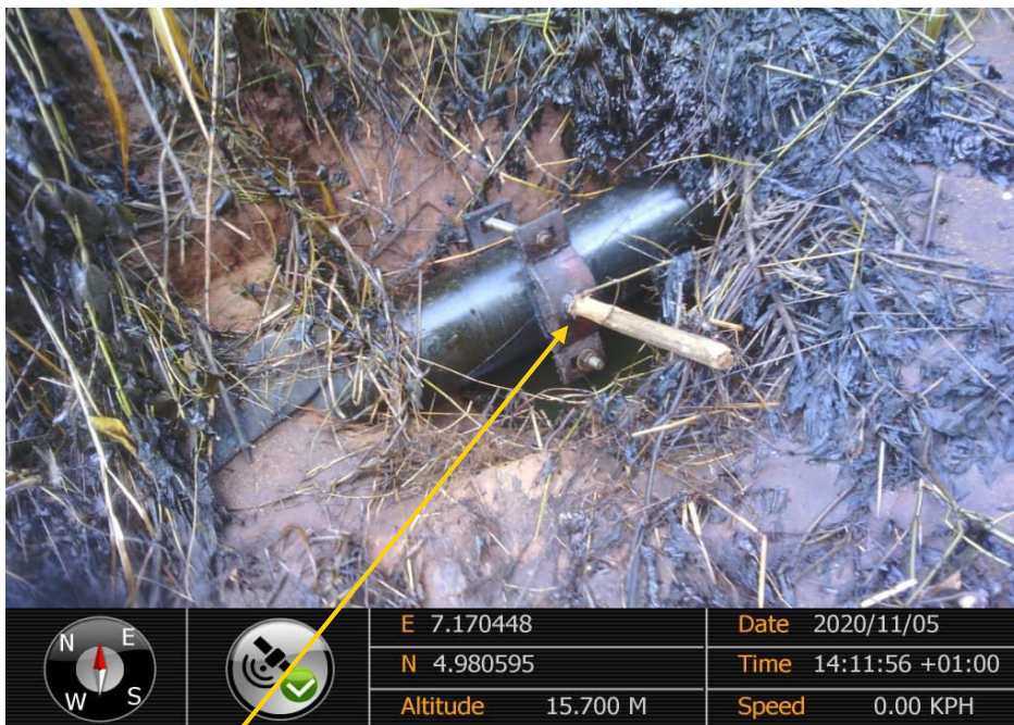
Close-up: Plugged drilled hole through a locally fabricated clamp at 2 o'clock position on 6'' Imoriver2 Imoriver1 bulkline at Odagwa . Picture was taken during Joint Investigation on 5th November 2020.
