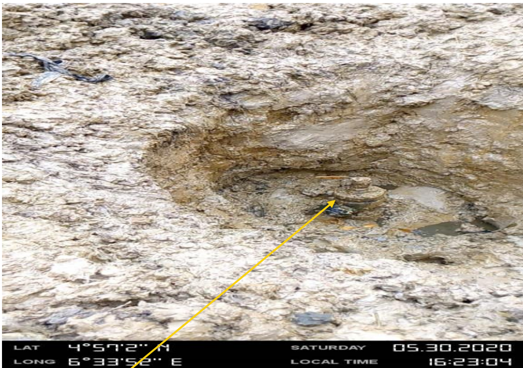
Close-up: 3'' ball valve illegal connection installed at 12 o'clock position on 20'' Kolocreek - Rumuekpe Pipeline at Aminigboko . Picture was taken during Joint Investigation 30th May 2020.
