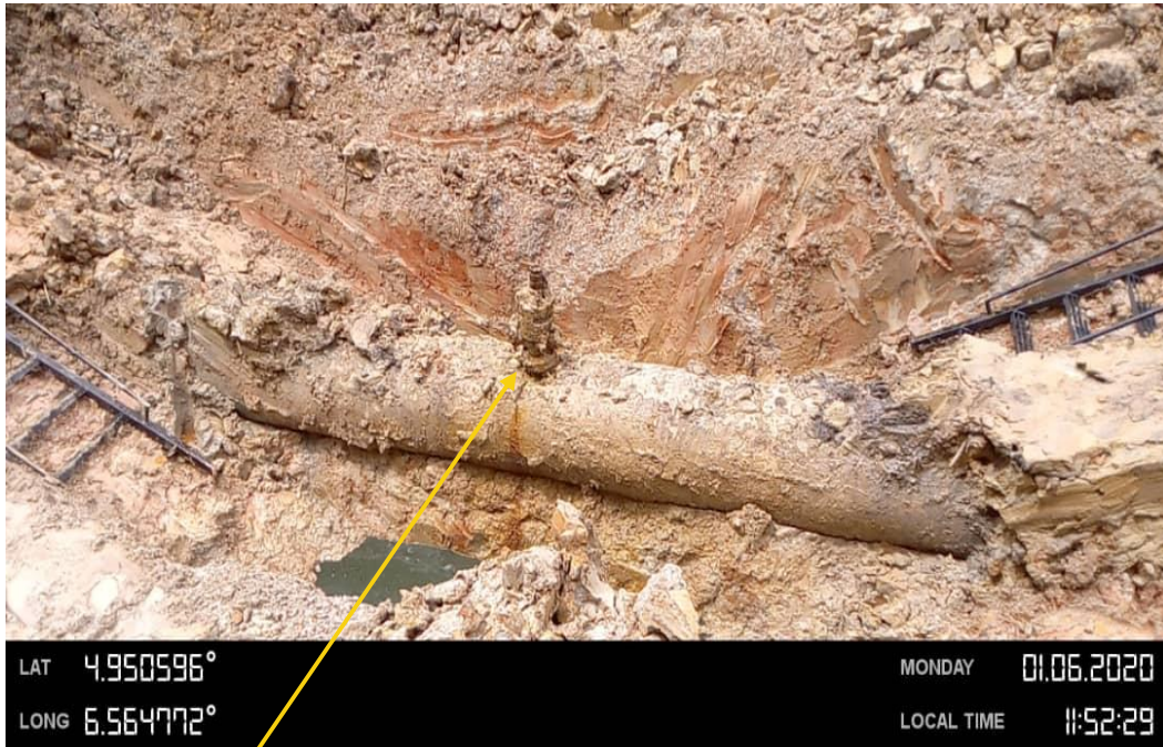
Close-up: 3" ball valve illegal connection installed at 12 o'clock position on 20" Kolocreek - Rumuekpe Pipeline at Aminigboko . Picture was taken on 1 st June 2020.
