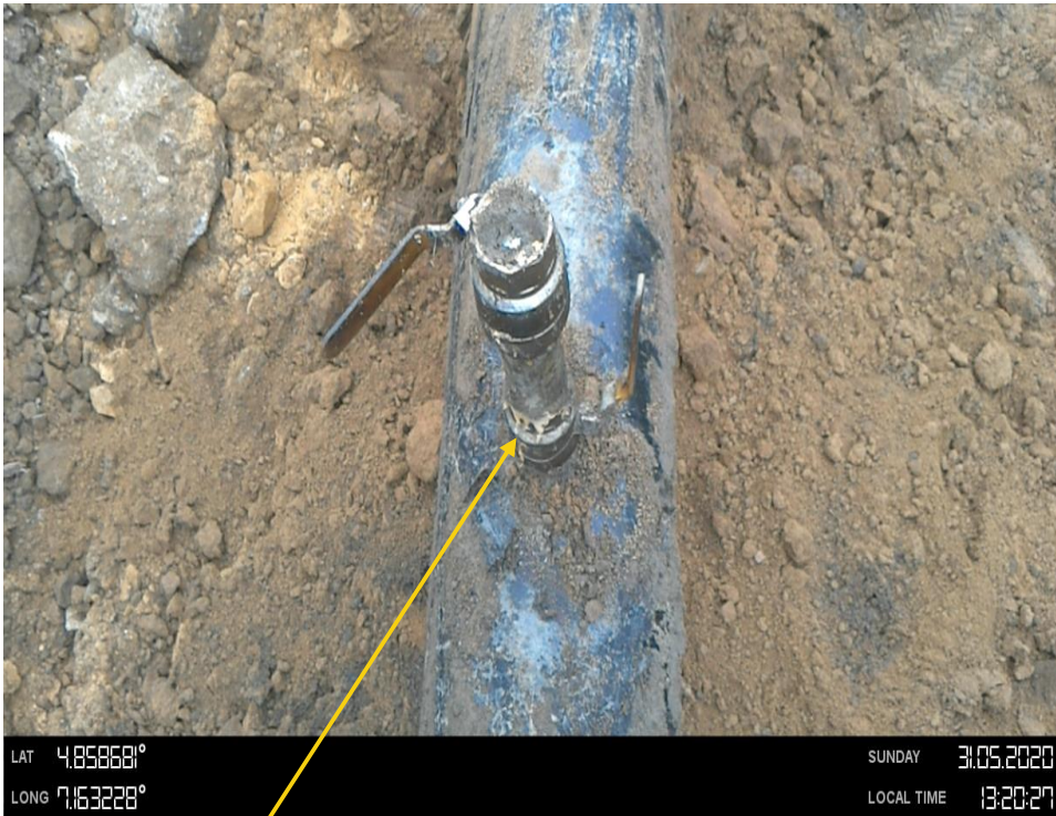
Close-up: Crude oil theft point installed at 12 o'clock position on 12" Imo River 2 Pipeline at Komkom. Picture was taken during Joint Investigation 30th May 2020.
