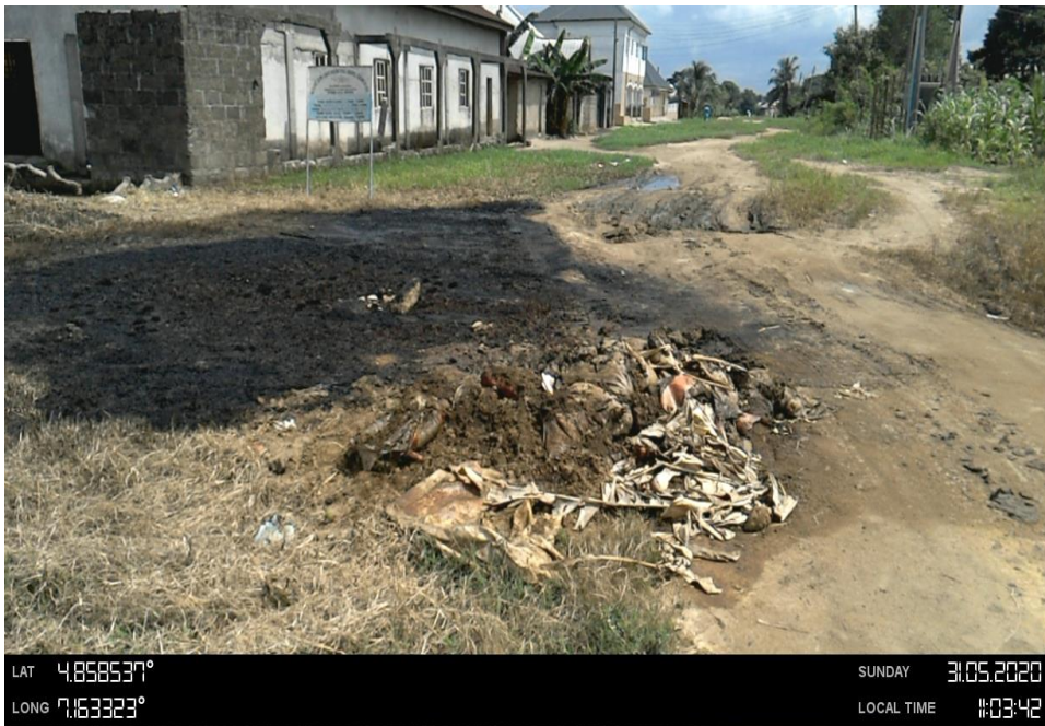
Overview: Part of spill impact on 12" Imo River 2 Pipeline at Komkom . Picture was taken during Joint Investigation 30th May 2020.
