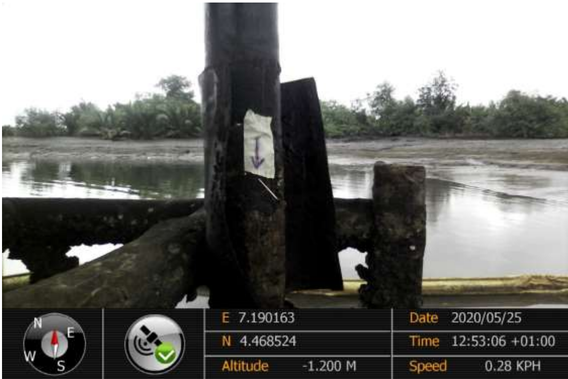
Overview 1: Part of spill impact on 4" Bonny Well 10s Flowline Riser at Oloma. Picture was taken during Joint Investigation 25th May 2020.
