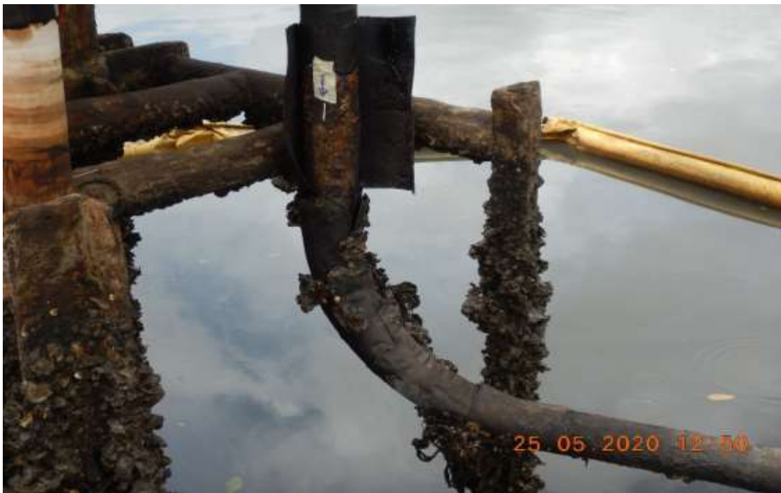
Close-up 2: Pin hole Leak on 4" Bonny Well 10s Flowline Riser at Oloma. Picture was taken during Joint Investigation 25th May 2020.
