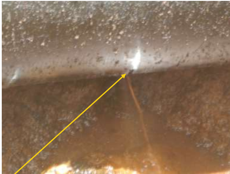
Close-up: Hacksaw cut at 6 o'clock position on 4" ImoRiver Well 55s Flowline at Igiriukwu. Picture was taken during Joint Investigation 5th May 2020.
