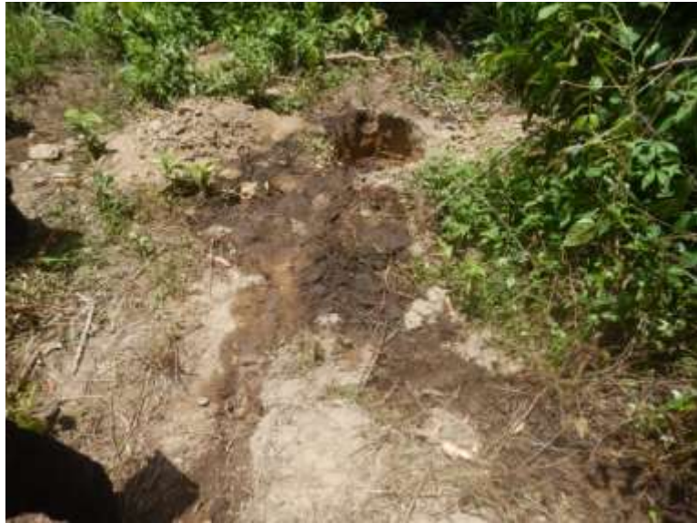
Overview: Part of spill impact on 4" ImoRiver Well 55s Flowline at Igiriukwu. Picture was taken during Joint Investigation 5th May 2020.
