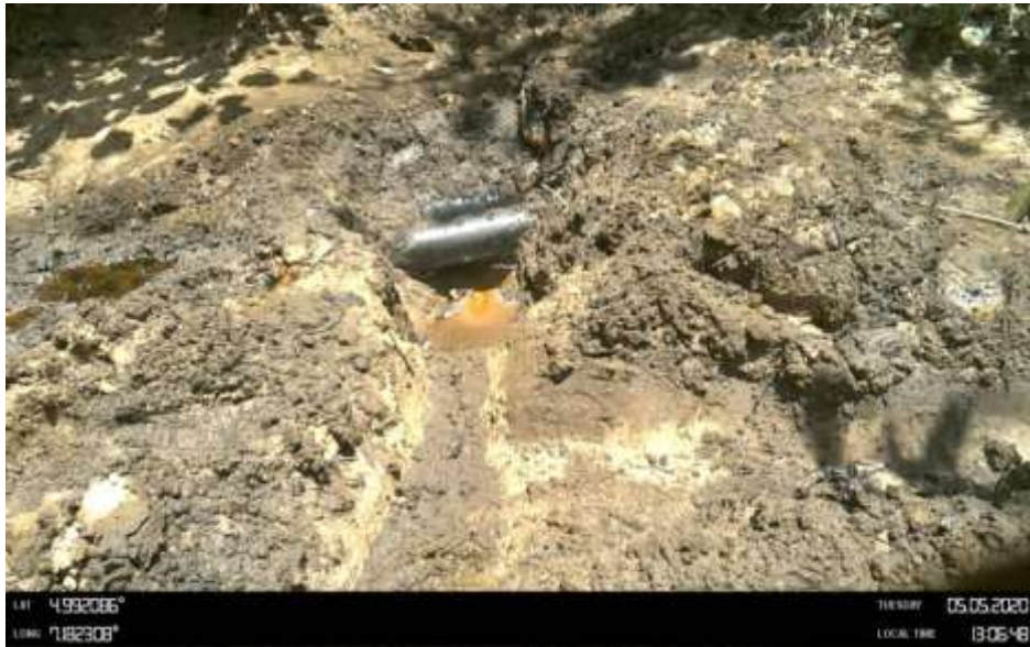
Overview: Part of spill impact on 4" ImoRiver Well 55s Flowline at Igiriukwu. Picture was taken during Joint Investigation 5th May 2020.
