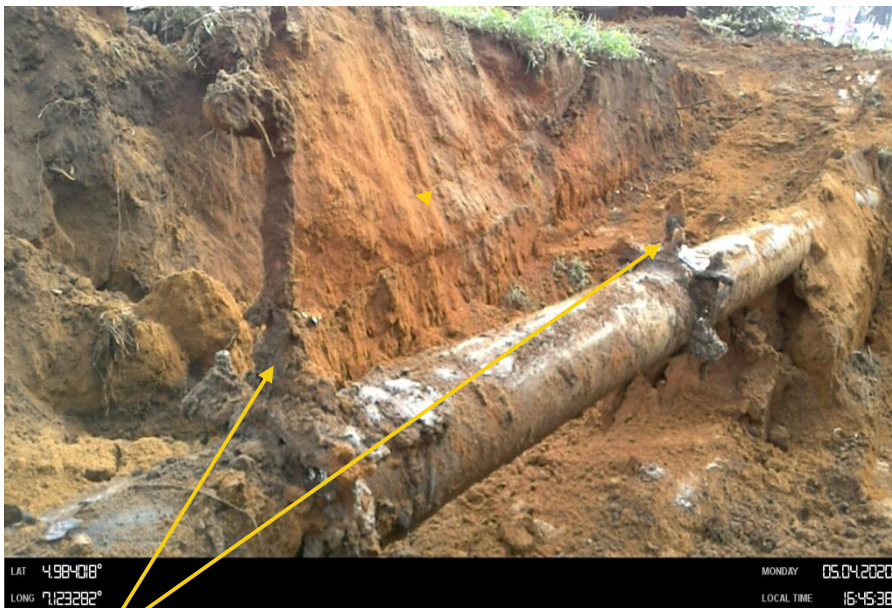
Close-up: 2 nos 1" valve crude oil theft points installed 1m apart at 12 o'clock position on 8" Nkali – ImoRiver2 Pipeline at Odagwa. Picture was taken during Joint Investigation of 4th May 2020.
