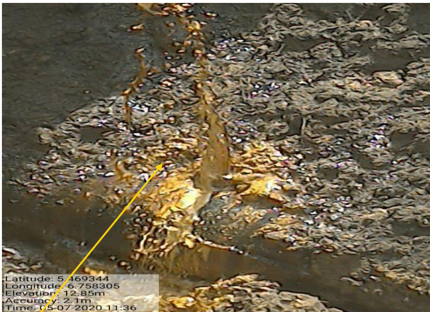
Close-up: 3" Nipple installed at 12 o'clock position on 16" Egbema Assa Pipeline at Etekwuru. Picture was taken during Joint Investigation of 7th May 2020.
