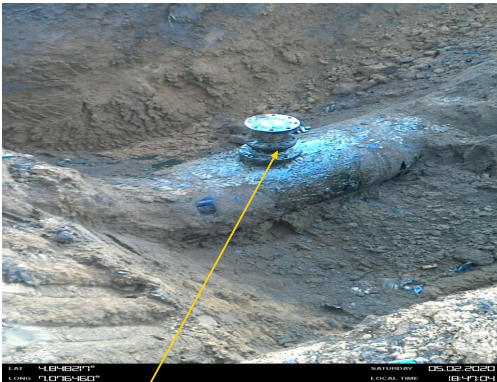
Close-up: 6" valve crude theft point installed at 12 o'clock position on on 28" Nkpoku Bomu Pipeline at Elenwo. Picture was taken during Joint Investigation of 2nd May 2020.
