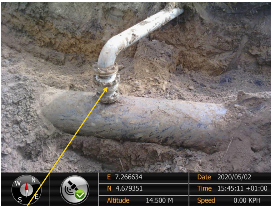
Close-up: 8" illegal valve connection at 12 o'clock position on 28" Nkpoku Bomu Pipeline at B-Dere. Picture was taken during Joint Investigation of 2 nd May 2020.
