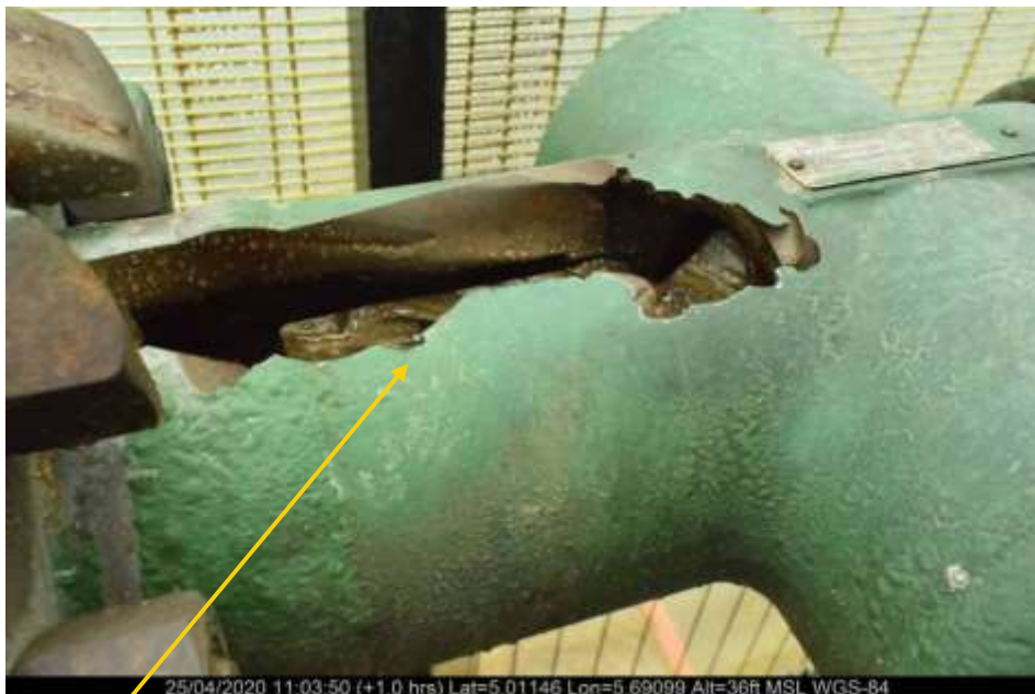
Close-up: Tear due to Internal erosion on 3" Well head on Well 24 Lima Bean Box at Ojobo. Picture was taken during Joint Investigation of 25 th April 2020.
