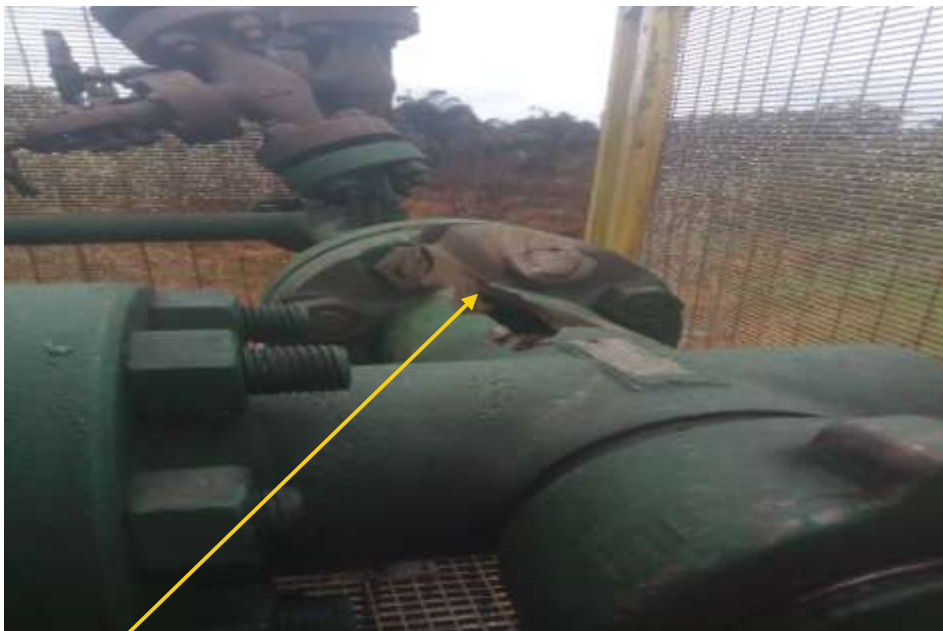
Close-up: Tear due to Internal erosion on 3" Well head on Well 24 Lima Bean Box at Ojobo. Picture was taken during Joint Investigation of 25 th April 2020
