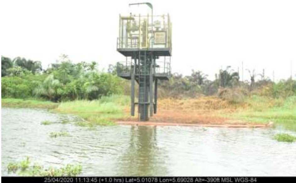
Overview: Part of spill impact on Well 24 Lima Bean Box at Ojobo. Picture was taken during Joint Investigation of 25 th April 2020.
