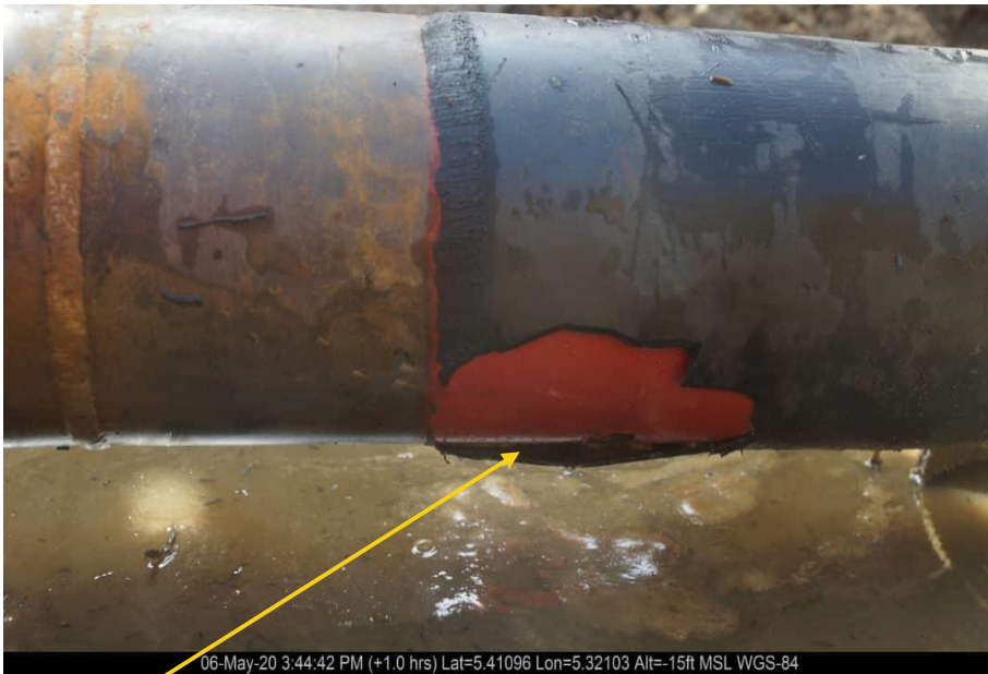
Close-up: Irregular hole at 7 o'clock position on 6" North bank central processing facility condensate delivery line at Obotobo. Picture was taken during Joint Investigation of 6th May 2020.
