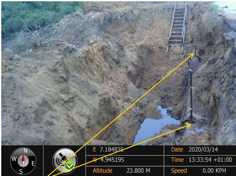
Close-up: 2 nos 1" valve installed 5m apart of crude oil at 12 o'clock position on 12" Imo River2 – Ogale Pipeline at Umulolo. Picture was taken during Joint Investigation of 14 th March 2020.
