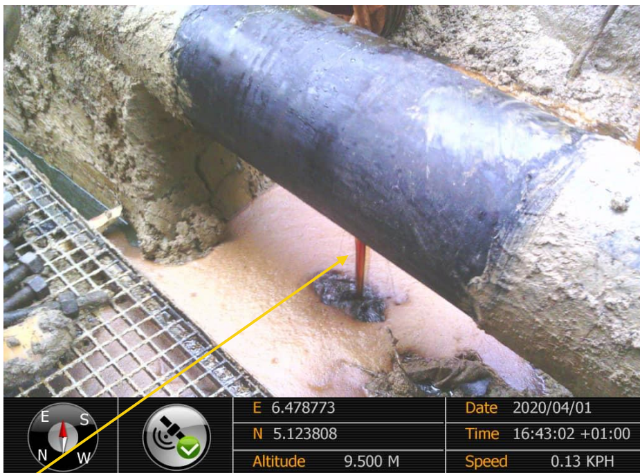
Close-up: 2cm Longitudinal Tear on 14" Okordia- Rumuekpe Pipeline at Akinima. Picture was taken during Joint Investigation of 1 st April 2020.
