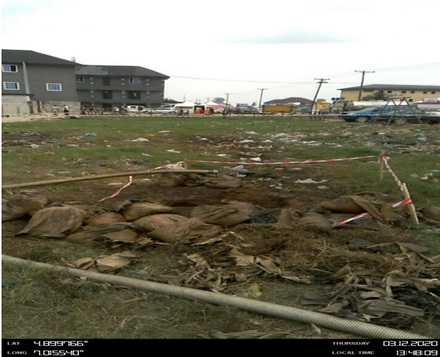
Overview: Part of spill impact on 28'' Nkpoku - Ebulu Pipeline at Rumuowha - Eneka. Picture was taken during Joint Investigation of 12 th March 2020.
