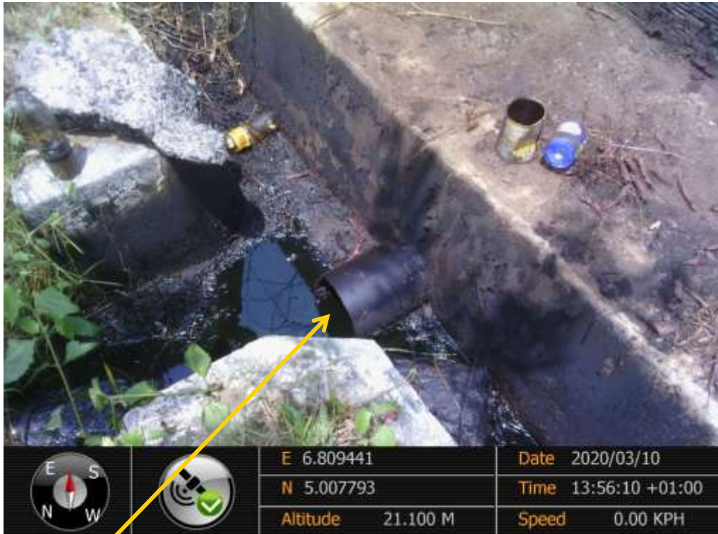
Close-up: Overflow from sewer-pit on Obele Flow station at Obele. Picture was taken during Joint Investigation of 10 th March 2020.
