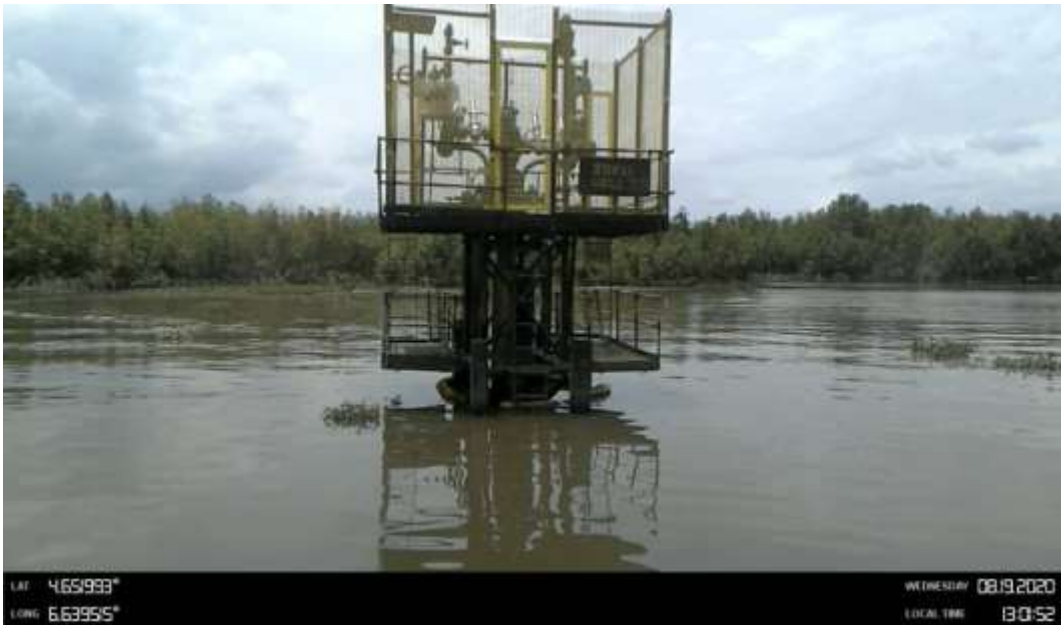
Overview: Part of spill impact on 4" Soku Well 23 Flowline at Ekineama 2. Picture was taken during Joint Investigation on 19th August 2020.
