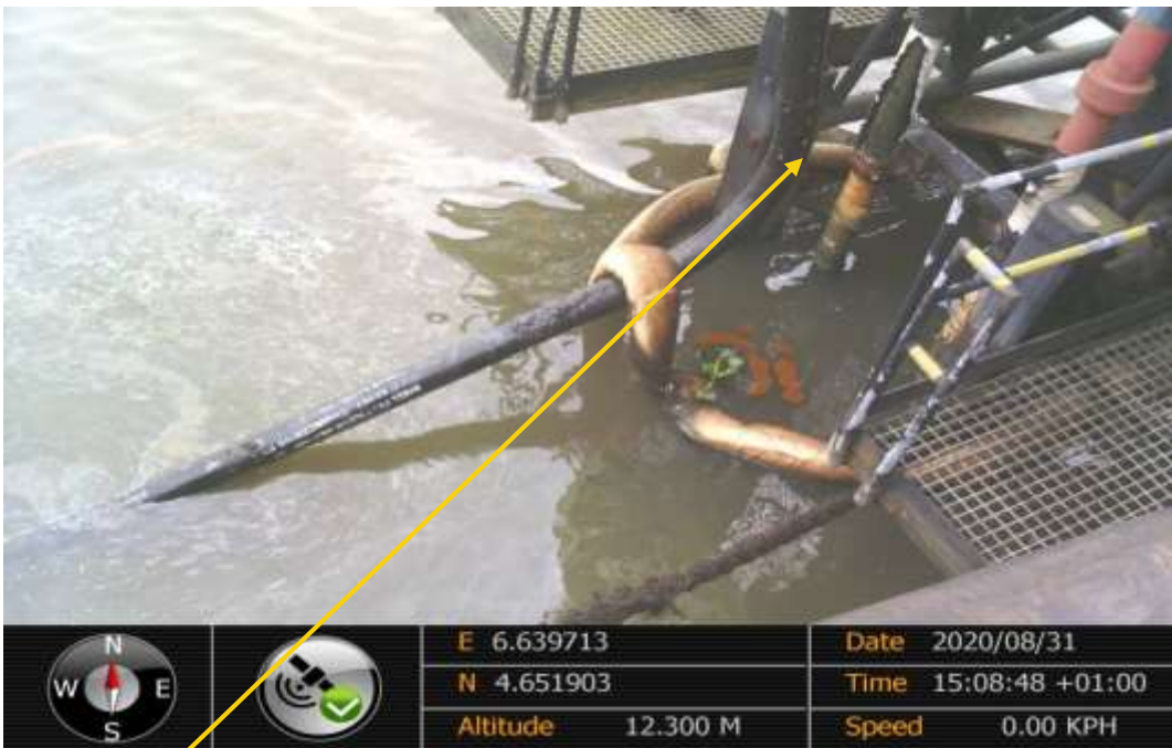
Close-up: Corrosion at 6 o'clock position on 4" Soku Well 23 Flowline at Ekineama 2. Picture was taken during Joint Investigation on 31st August 2020.
