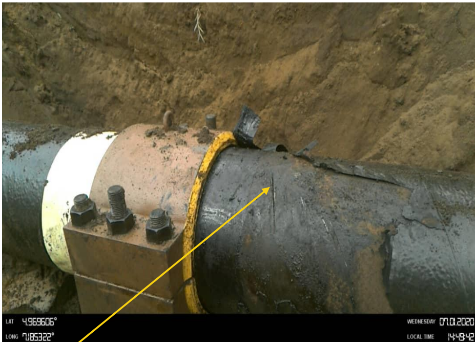
Close-up: 5cm Hacksaw cut from a 12 o'clock to 3 o'clock position on 12" ImoRiver - Ogale Pipeline at Umulolo. Picture was taken during Joint Investigation 1st July 2020.
