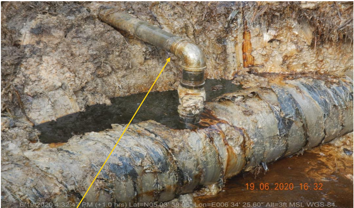
Closeup 1: Crude Oil theft point installed at 12 o'clock position on 14" Okordia Rumuekpe Pipeline at Ula-Okobo. Picture was taken during Joint Investigation 19th June 2020.
