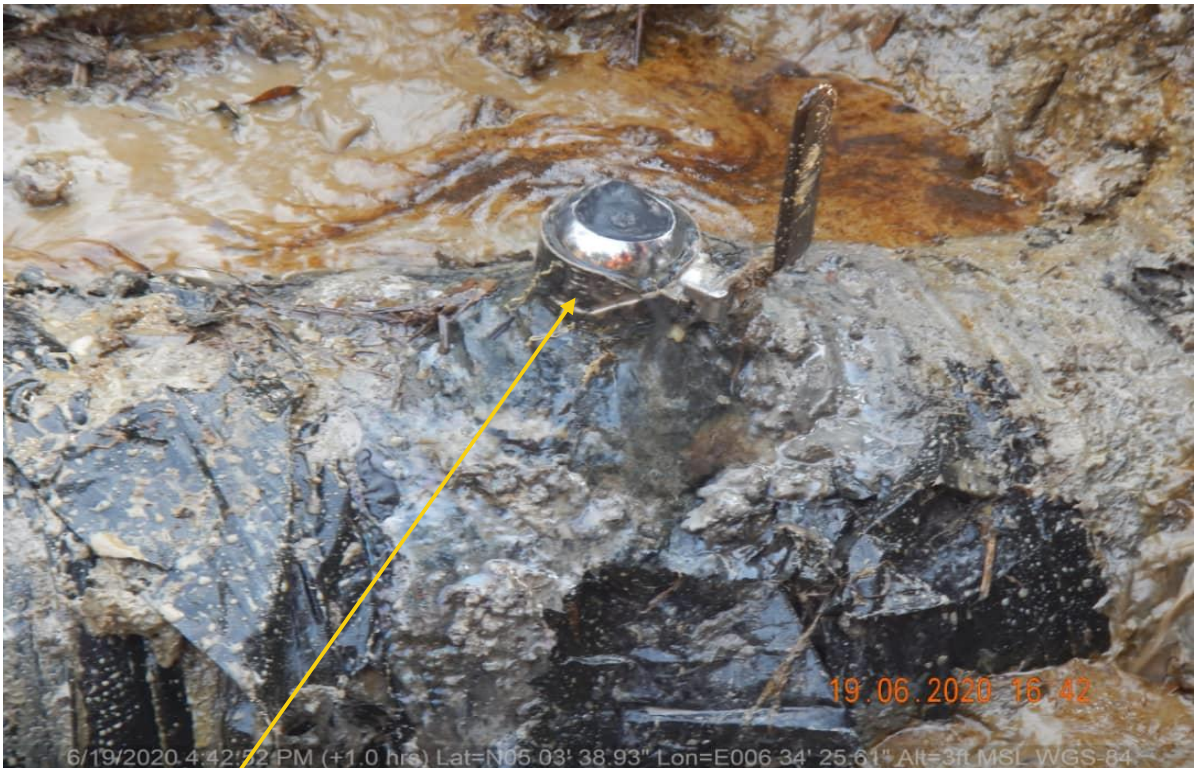
Close-up 2: Crude Oil theft point installed at 12 o'clock position on 14" Okordia Rumuekpe Pipeline at Ula-Okobo. Picture was taken during Joint Investigation 19th June 2020.
