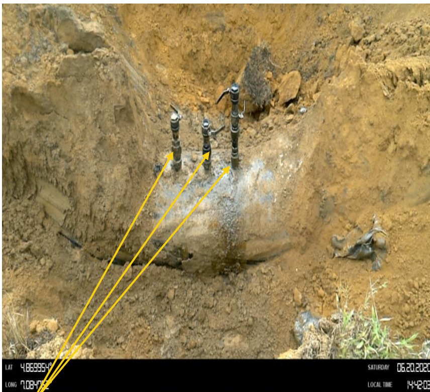
Close-up: 3 nos 3" bulb valves installed at 12 o'clock position on 36" Nkpoku - Ogale Pipeline at Rumuokwursi. Picture was taken during Joint Investigation 20th June 2020.
