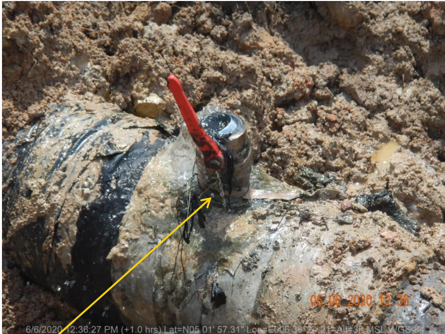
Close-up: Crude oil theft point installed at 12 o'clock position on 14" Okordia - Rumuekpe Pipeline at Edeoha. Picture was taken during Joint Investigation of 6 th June 2020
