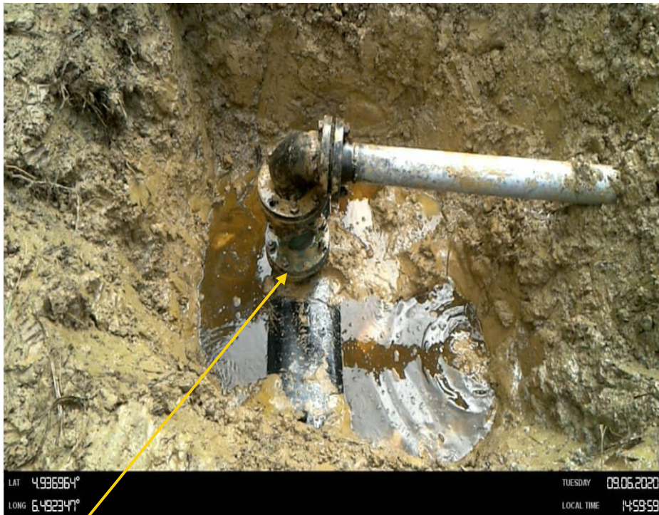
Close-up: 4" ball valve installed at 12 o'clock position on New 20" Kolocreek - Rumuekpe Pipeline at Odau KP15.3 . Picture was taken during Joint Investigation 9th June 2020.
