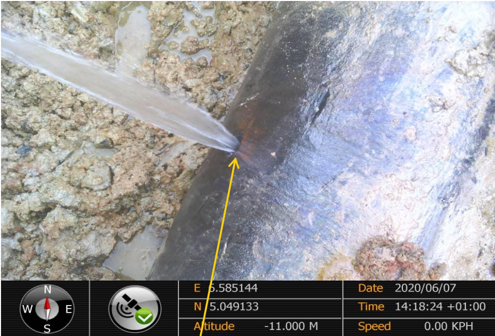
Close-up: 2 of 2nos of smooth round-edge holes on 14" Okordia - Rumuekpe Pipeline at Ula-Ikata. Picture was taken during Joint Investigation of 7 th June 2020
