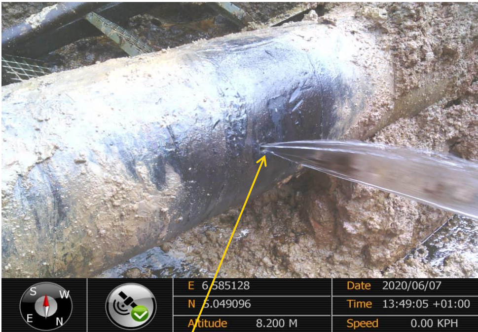
Close-up: 1 of 2nos of smooth round-edge holes on 14" Okordia - Rumuekpe Pipeline at Ula-Ikata. Picture was taken during Joint Investigation of 7 th June 2020
