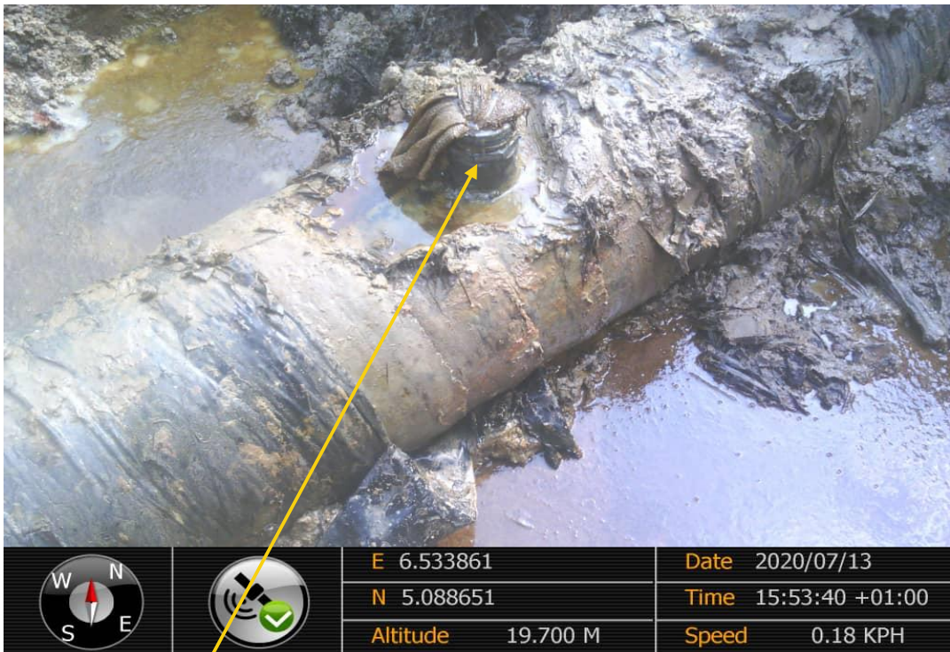
Close-up: Crude oil theft point installed at 12 o'clock position on 14" Okordia Rumuekpe Pipeline at Ukpeliède. Picture was taken during Joint Investigation on 13th July 2020.
