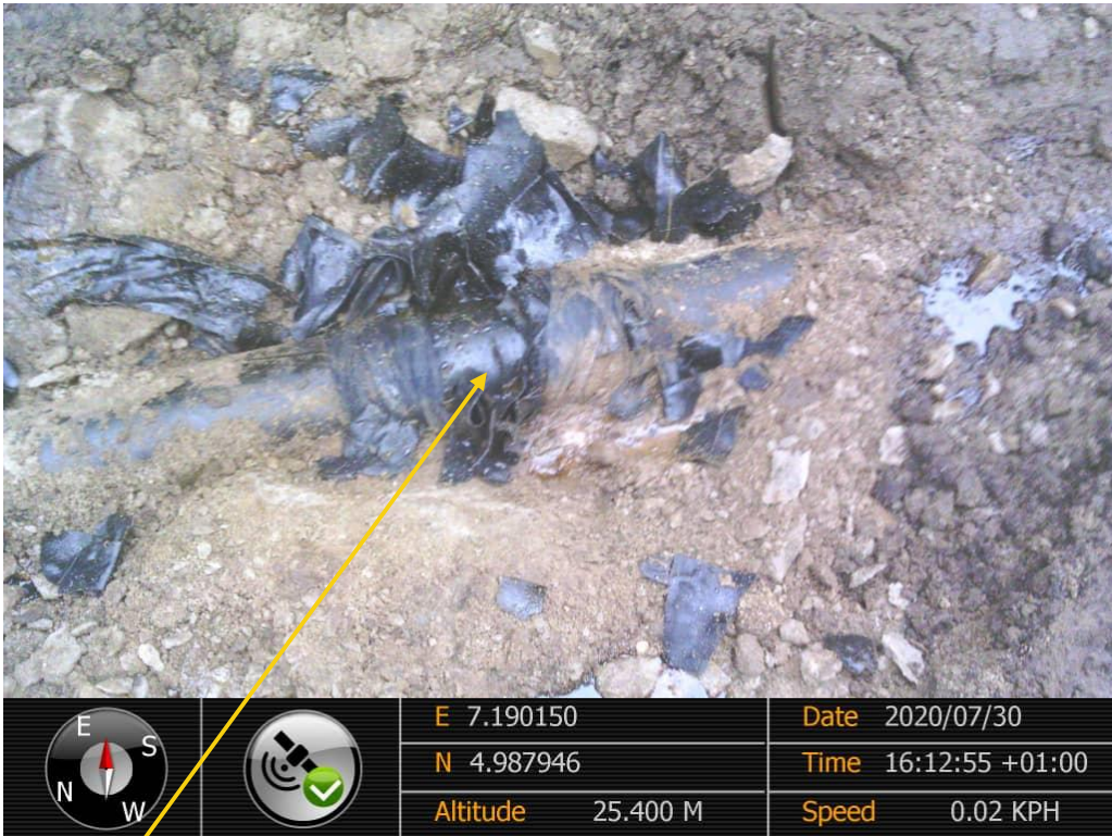
Close-up: Hack Saw Cut on 4" Imo River Well 32L Flowline at Igiriukwu-Owaza. Picture was taken during Joint Investigation of 30 th July 2020.
