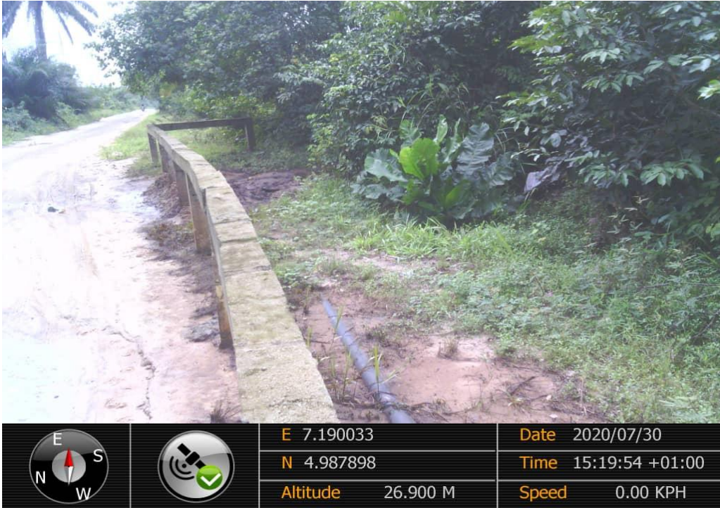
Overview: Part of spill impact on 4" Imo River Well 32L Flowline at Igiriukwu-Owaza. Picture was taken during Joint Investigation of 30 th July 2020.
