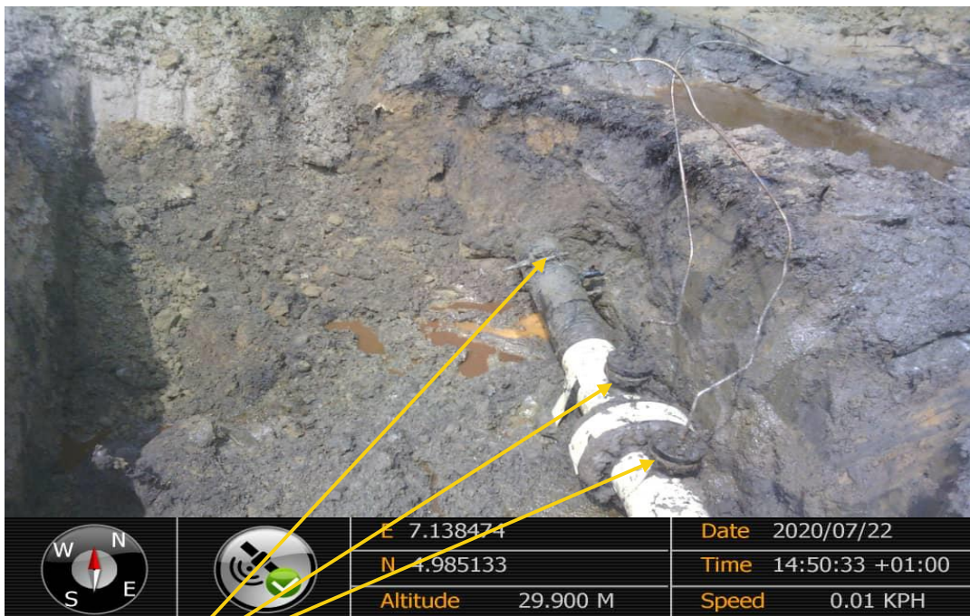
Close-up: 1" Locally fabricated clamp installed alongside with 1" valve at 12 o'clock position on 8" Nkali - ImoRiver 2 Pipeline at Odagwa. Picture was taken during Joint Investigation on 22nd July 2020.
