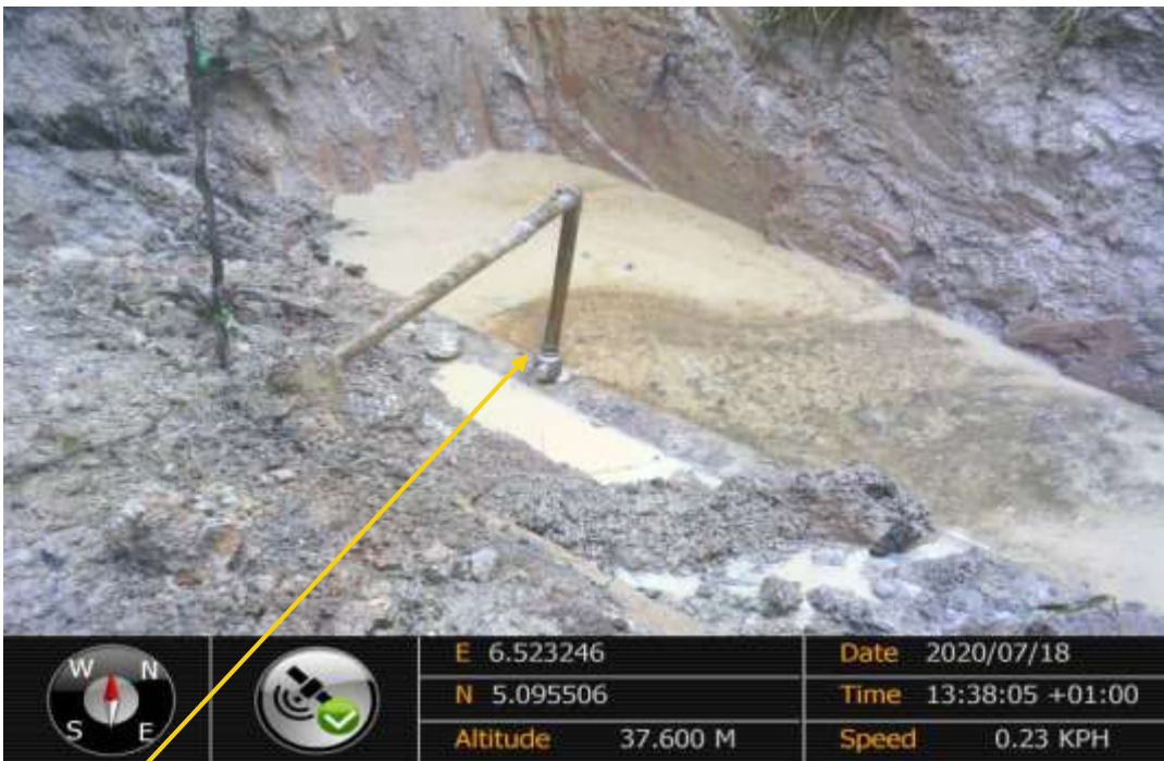
Close-up: Failed 2inch ball valve fittings installed at 12 o'clock position on 14" Okordia Rumuekpe Pipeline at Idu-Ekpeye . Picture was taken during Joint Investigation 18th July 2020.
