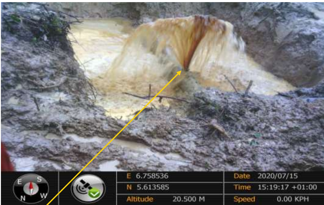
Close-up: 4inch valve installed at 12 o'clock position on 12" Oguta Assa Pipeline at Opuoma Picture was taken during Joint Investigation 15th July 2020.
