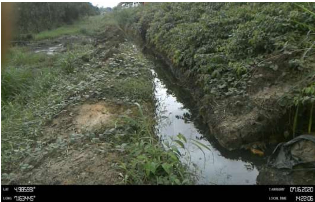
Overview: Part of spill impact on 8" Nkali Ogale Pipeline at Odagwa. Picture was taken during Joint Investigation 16th July 2020.
