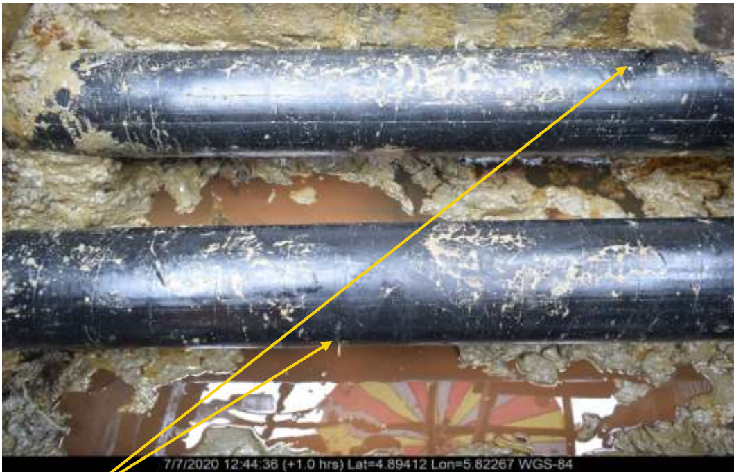
Close-up 1: Hack saw cut at 3'o clock position and 9 o'clock position on 8" Seibou-Ajatiton Bulklineat Agbidiamma. Picture was taken during Joint Investigation 7th July 2020.
