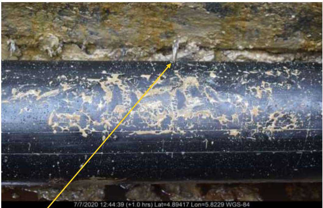
Close-up 3: Hack saw cut at 3'o clock position and 9 o'clock position on 8" Seibou-Ajatiton Bulklineat Agbidiaama. Picture was taken during Joint Investigation 7th July 2020
