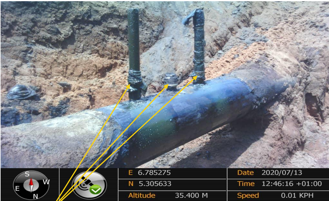
Close-up: 3nos 2" Ball valves installed at 12 o'clock position on 18" Assa - Rumuekpe Pipeline at Awara. Picture was taken during Joint Investigation 13th July 2020.
