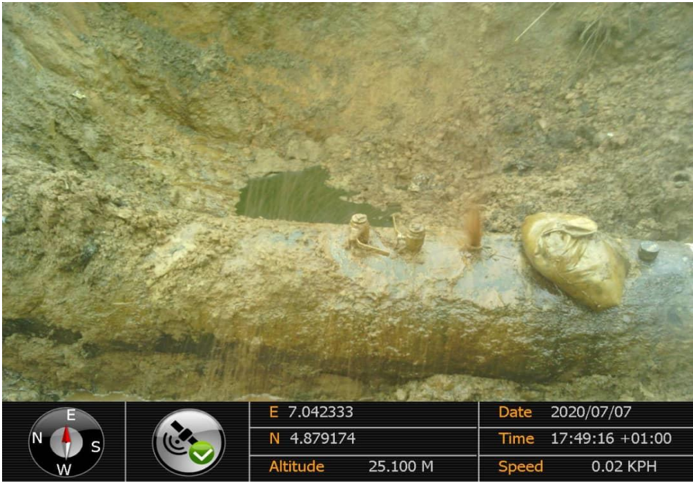
Close-up: 5nos 2'' Illegal connections installed 12 o'clock position on 28'' Nkpoku Bomu Pipeline at Rumuewhara . Picture was taken during Joint Investigation 7th July 2020.
