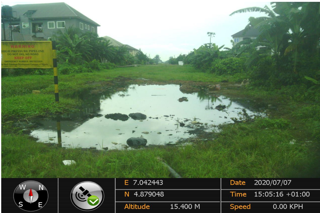
Overview: Part of spill impact on 28" Nkpoku Bomu Pipeline at Rumuewhara . Picture was taken during Joint Investigation 7th July 2020.
