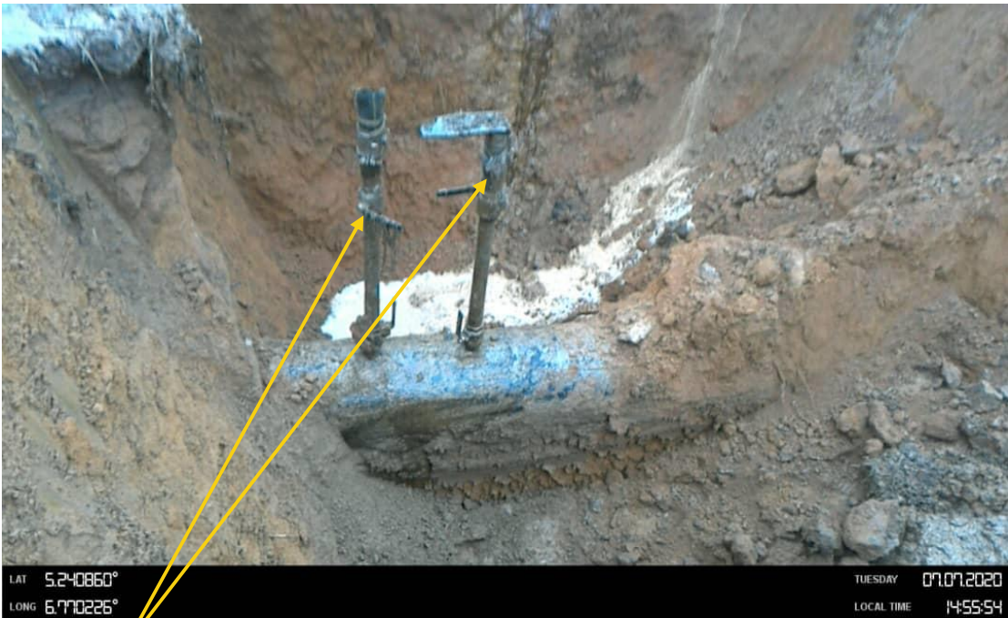
Close-up: 2nos Ball valves installed at 12 o'clock position on 18" Assa - Rumuekpe Pipeline at Egbeda. Picture was taken during Joint Investigation 7th July 2020.
