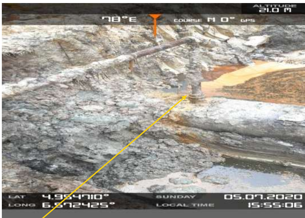
Close-up: Failed 3" Ball valve fittings installed at 12 o'clock position on 20" Kolocreek – rumuekpe Pipeline at Owerewere . Picture was taken during Joint Investigation 5th July 2020.
