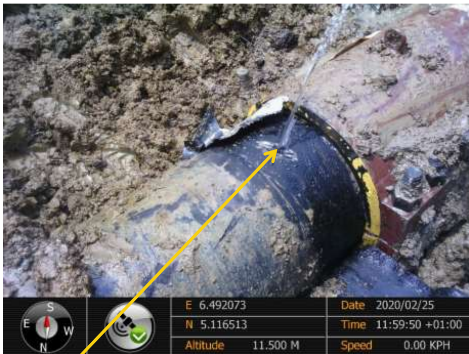
Close-up: Point 3 drilled hole at 12 o'clock position on 14" Okordia Rumuekpe Pipeline showing water and oil at Akalamini. Picture was taken during Joint Investigation of 25 th February 2020.
