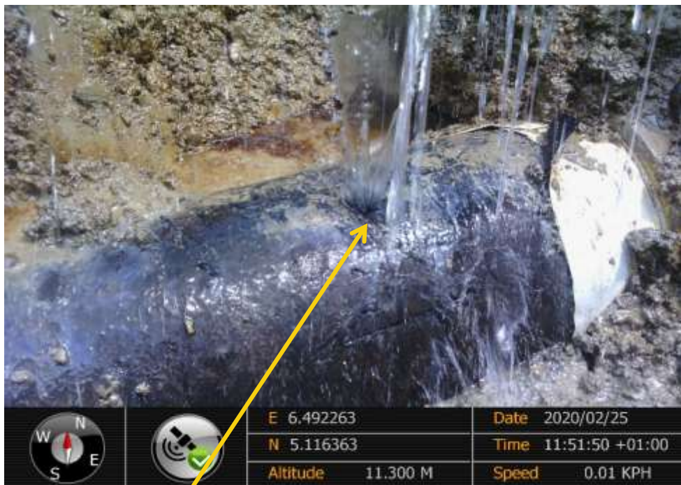
Close-up: Point 1 drilled hole at 12 o'clock position showing water and oil on 14" Okordia Rumuekpe Pipeline at Akalamini. Picture was taken during Joint Investigation of 25 th February 2020.
