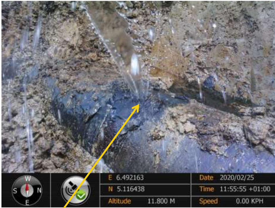
Close-up: Point 2 drilled hole at 12 o'clock position on 14" Okordia Rumuekpe Pipeline showing water and oil at Akalamini. Picture was taken during Joint Investigation of 25 th February 2020.
