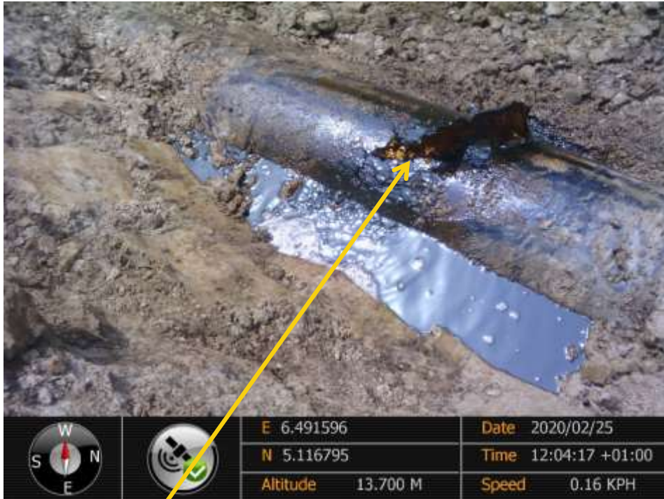
Closeup: Point 4 drilled hole at 12 o'clock position on 14" Okordia Rumuekpe Pipeline at Akalamini. Picture was taken during Joint Investigation of 25 th February 2020.
