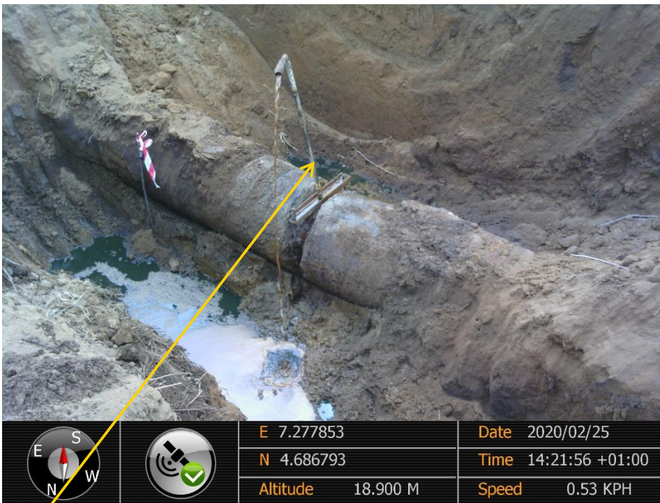
Close-up: 1" valve installed at at 12 o'clock position on 24" Ogale – Bomu Pipeline at Biara . Picture was taken during Joint Investigation of 25 th February 2020.
