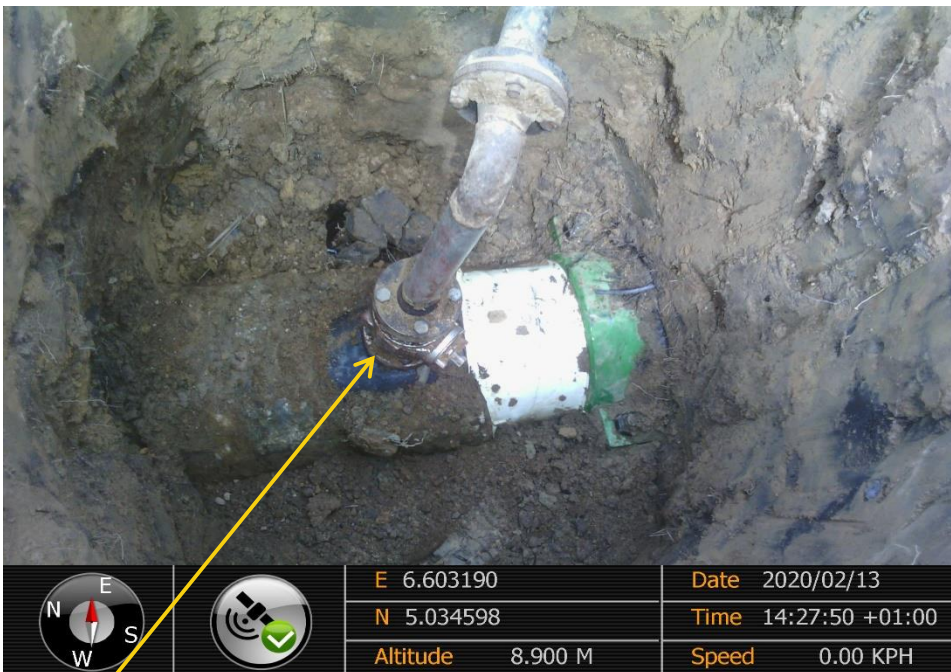
Close-up: Crude oil theft point installed at 12 o'clock position on 14" Okordia - Rumuekpe Pipeline at Ikata. Picture was taken during Joint Investigation of 13 th February 2020.
