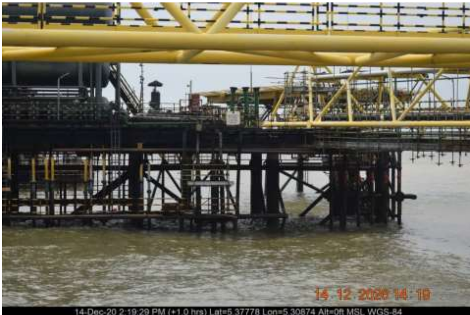
Close-up: External Corrosion at 3 o'clock on 12inch Forcados low pressure delivery line at Ogulagha. Picture was taken during Joint Investigation of 14 th December 2020
