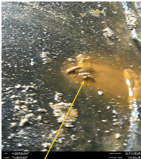
Close-up 1: 4 nos 5mm drilled hole (leak point 1) at 10 o'clock position on 36inch Nkpoku Ogale Pipeline at Agbonchia. Picture was taken during Joint Investigation on 17th Dec 2020.
