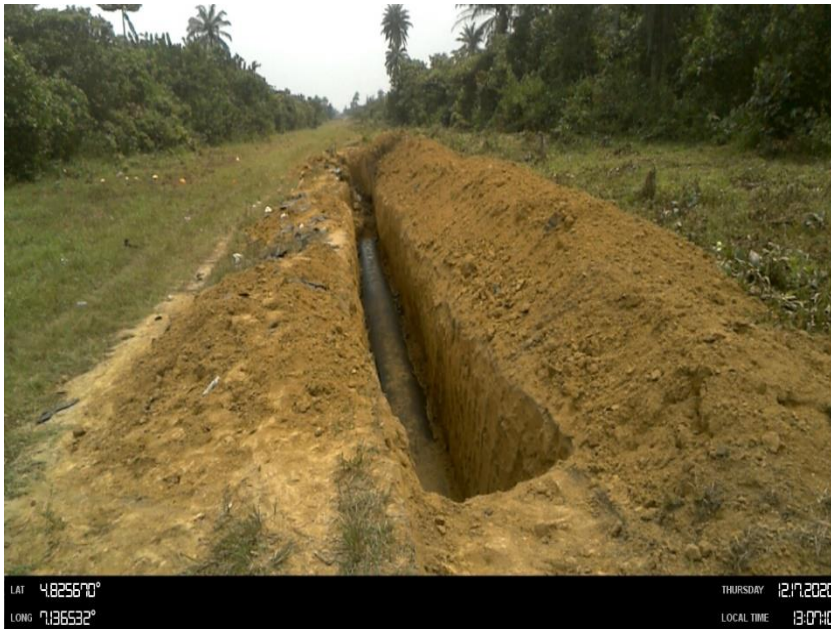
Overview: Part of spill impact on 36'' Nkpoku Ogale Pipeline at Agbonchia. Picture was taken during Joint Investigation on 17th Dec 2020.
