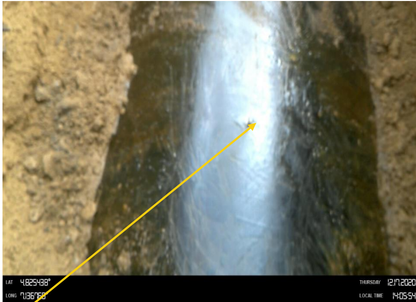
Close-up 4: 4 nos 5mm drilled hole (leak point 3) at 12 o'clock position on 36inch Nkpoku Ogale Pipeline at Agbonchia. Picture was taken during Joint Investigation on 17th Dec 2020.
