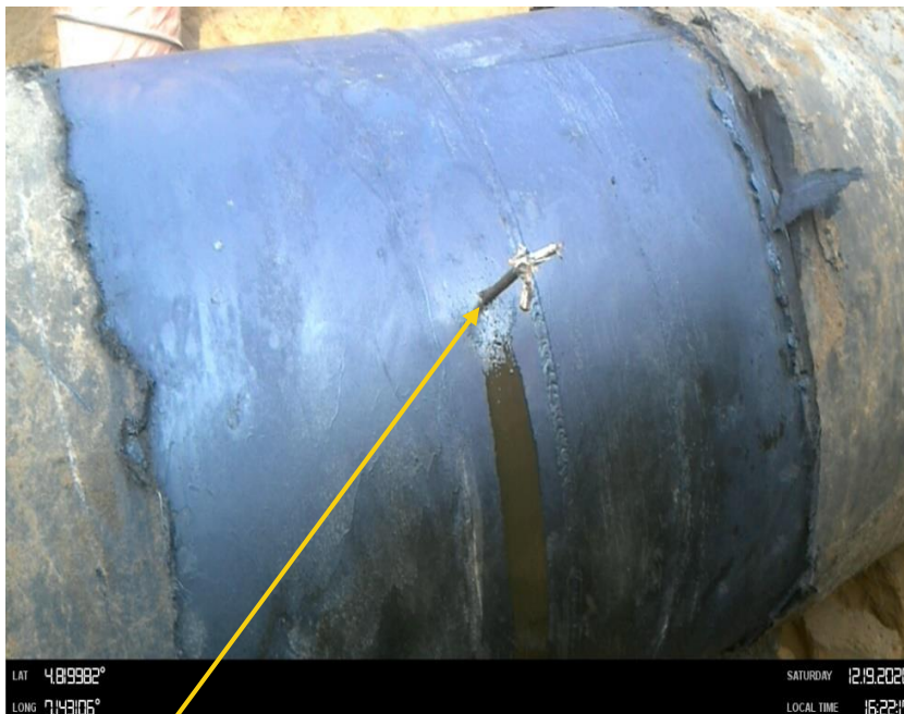
Close-up: Plugged 5mm Drilled hole at 2 o'clock position on 36" Nkpoku Ogale Pipeline at Ogale. Picture was taken during Joint Investigation on 19th Dec 2020.
