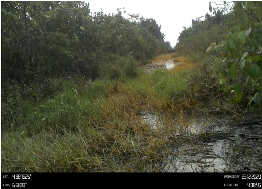
Overview: Part of spill impact on 20'' Kolocreek Rumuekpe Pipeine at Owerewere. Picture was taken during Joint Investigation on 23rd Dec 2020.
