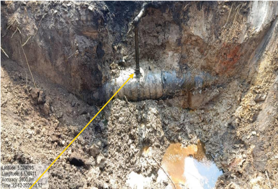
Close-up: 2" valve installed at 12 o'clock position connected to a 2" galvanized pipe on 14" Okordia Rumuekpe Pipeine at Edeoha. Picture was taken during Joint Investigation on 22nd Dec 2020.
