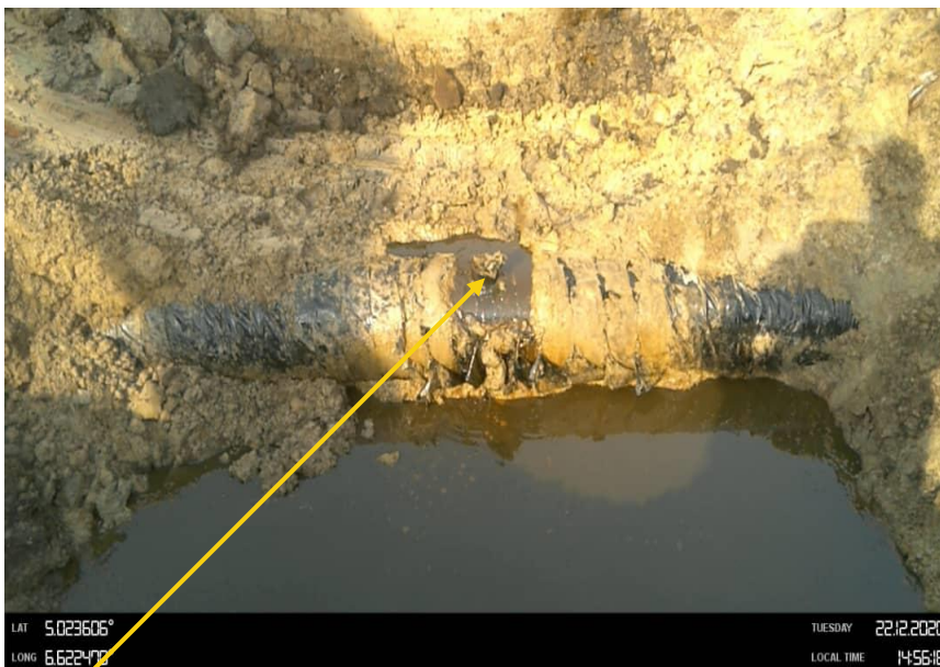
Close-up: 3" nipple installed at 12 o'clock position on 14" Okordia Rumuekpe Pipeine at Edeoha. Picture was taken during Joint Investigation on 22nd Dec 2020.
