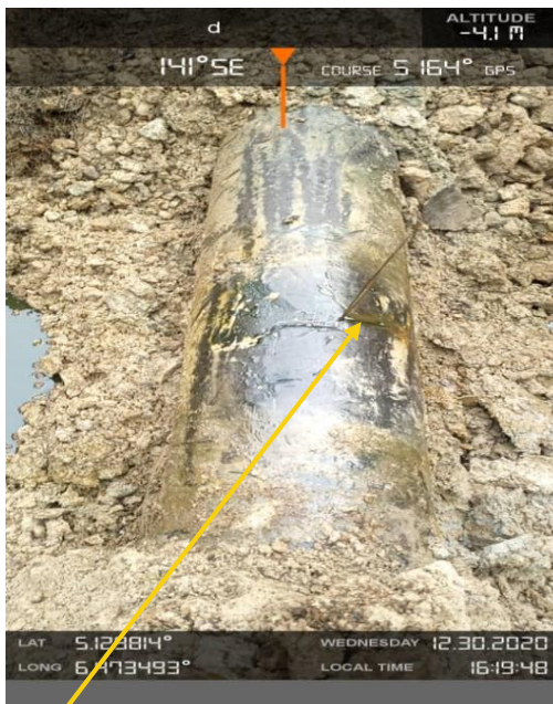
Close-up: Hack Saw Cut at 12:30 o'clock position on 14" Okordia Rumuekpe Pipeine at Akinima. Picture was taken during Joint Investigation on 30 th December 2020.
