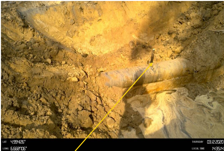
Close-up: Plugged 3inch nipple installed at 12 o'clock position on 14inch Okordia Rumuekpe Pipeline at Rumuekpe (Imogu). Picture was taken during Joint Investigation on 3rd December 2020.
