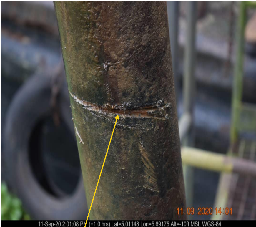
Close-up: Hacksaw cut on 4" Benisese well 16T Flowline at Ojobo Picture was taken during Joint Investigation on 11th September 2020.
