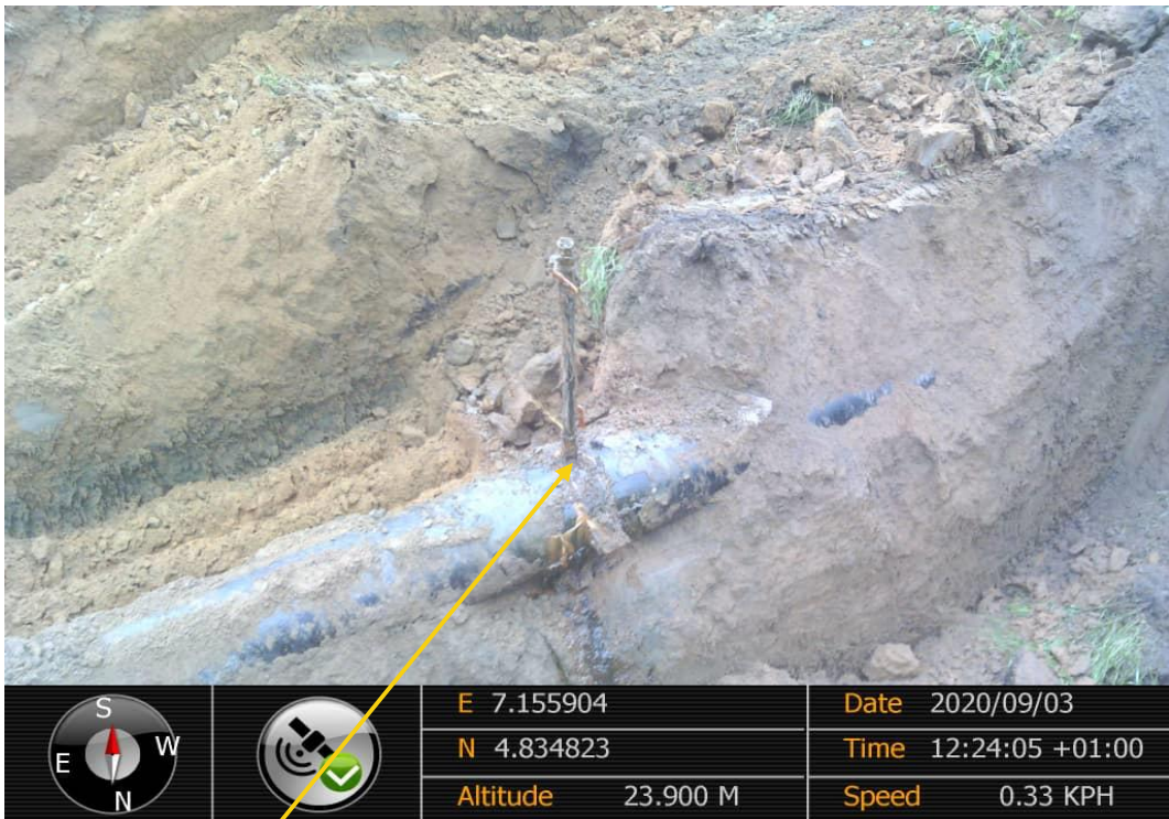
Close-up: Crude oil theft point installed at 12 o'clock position on 12" ImoRiver1- Ogale Pipeline at Ogale. Picture was taken during Joint Investigation on 3rd September 2020.
