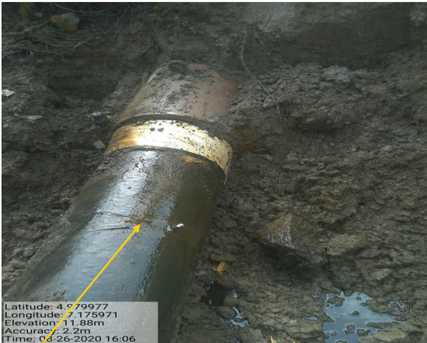
Close-up: Hacksaw cut at 11 o'clock position on 12" ImoRiver2- Ogale Pipeline at Igiriukwu-Isietitioha Owaza. Picture was taken during Joint Investigation on 26th August 2020.
