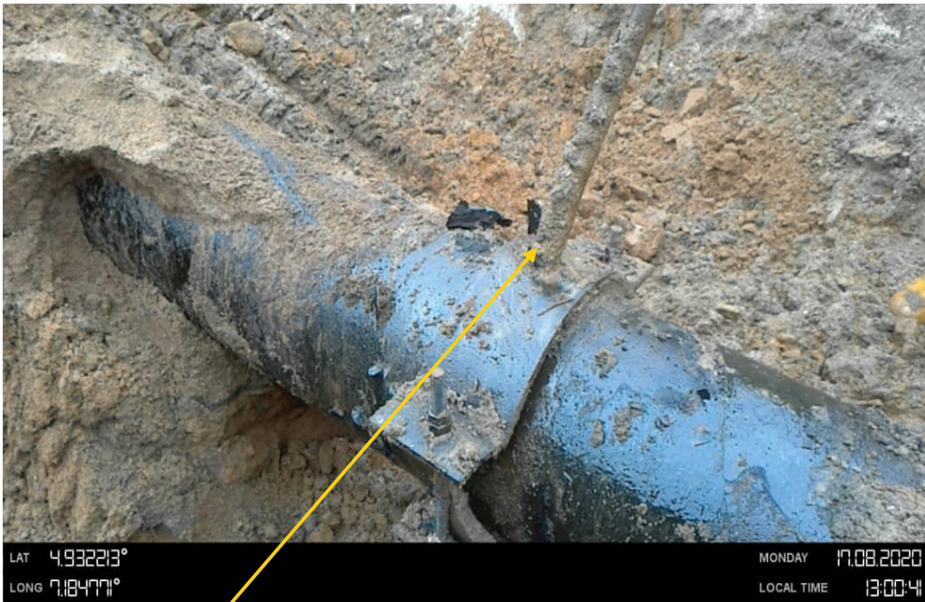
Close-up: Crude theft point installed at 12 o'clock position on 12" ImoRiver1 - Ogale Pipeline at Okohia. Picture was taken during Joint Investigation 17 th August 2020.
