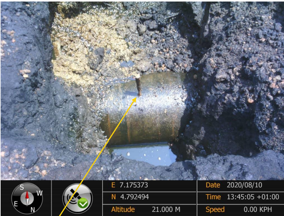
Close-up: Plugged drilled hole of 1cm diameter installed at 12 o'clock position on 24" Nkpoku Bomu Pipeline at Egbalor. Picture was taken during Joint Investigation 10th August 2020.
