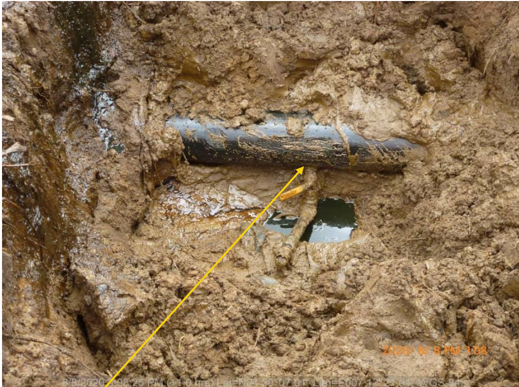
Close-up: Crude oil theft point installed at 7 o'clock position on 6" Imo River Well 59T Flowline at Igiriukwu-Owaza. Picture was taken during Joint Investigation of 8 th August 2020.
